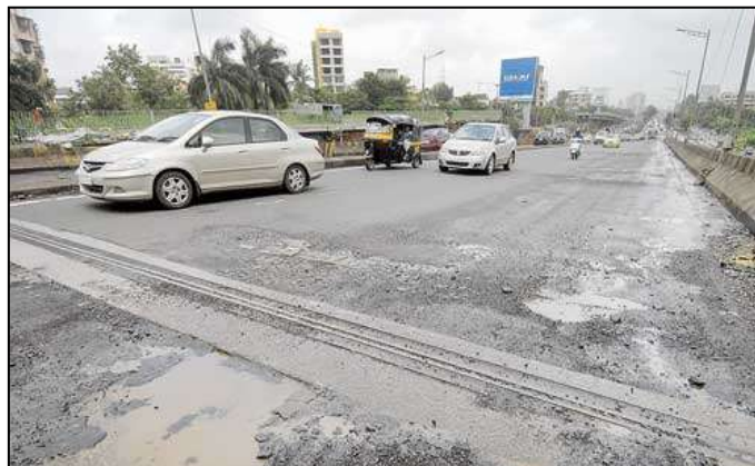
Poorly maintained Western Express Highway
