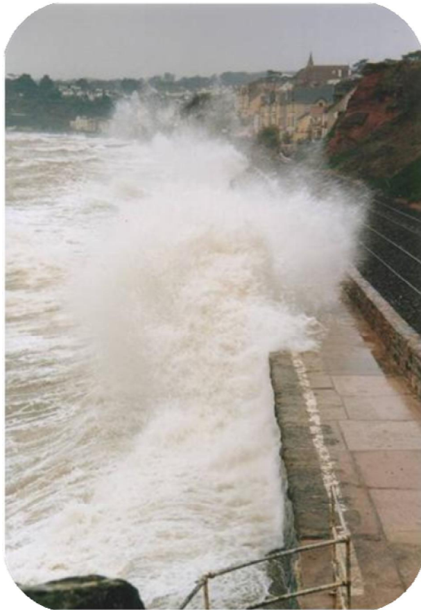
Figure 4-7 Wave Overtopping Dawlish
