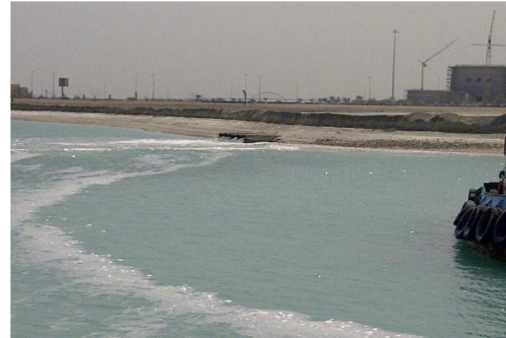
Figure 4-18 Pollution Control Via Silt boxes Bahrain
