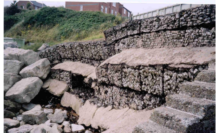
Figure 4-14 Failed Gabion Baskets, Poole, Southern England
